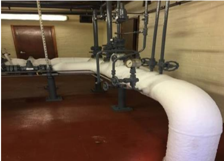
Figure 10 : ice forming following failure of heating asset.
