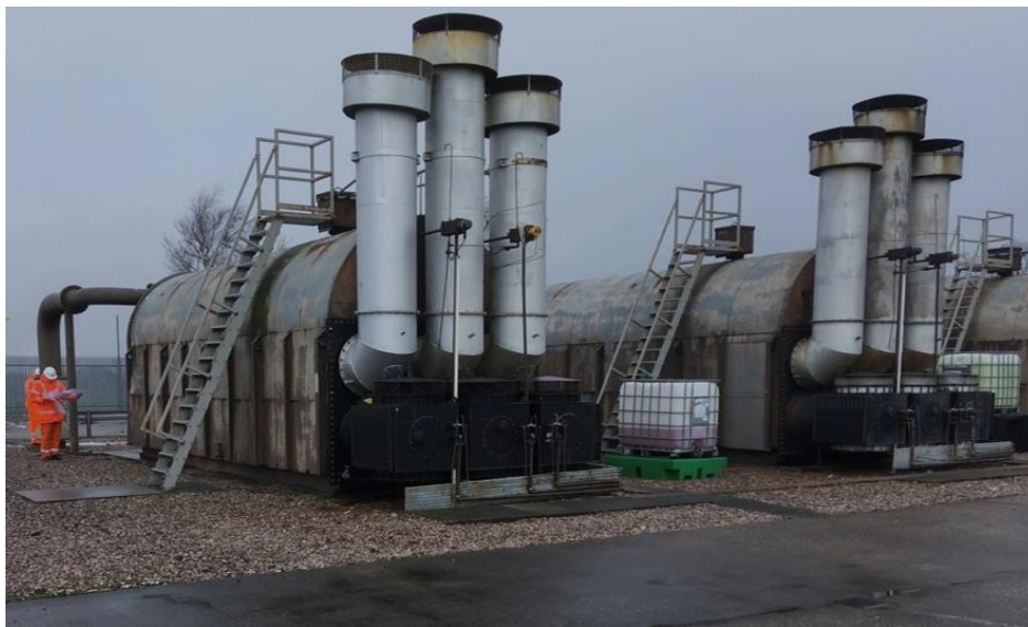
Figure 2 – Water bath heaters.
