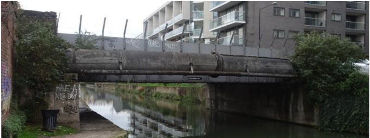
Figure 4: Bow Common Lane pipeline crossing condition at initial inspection
