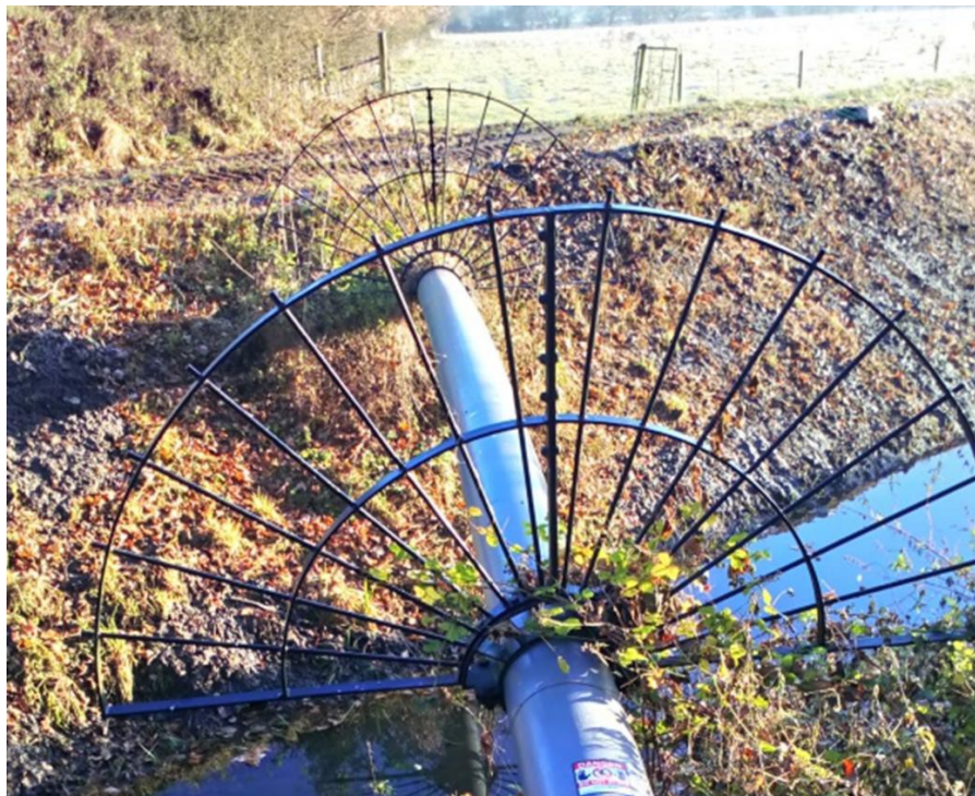
Figure A2: Example of Fans and anti-vandal guards
