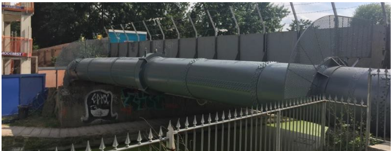
Figure 5: Bow Common Lane pipeline crossing condition after pipe remediation and fitting of new access deterrent measure
