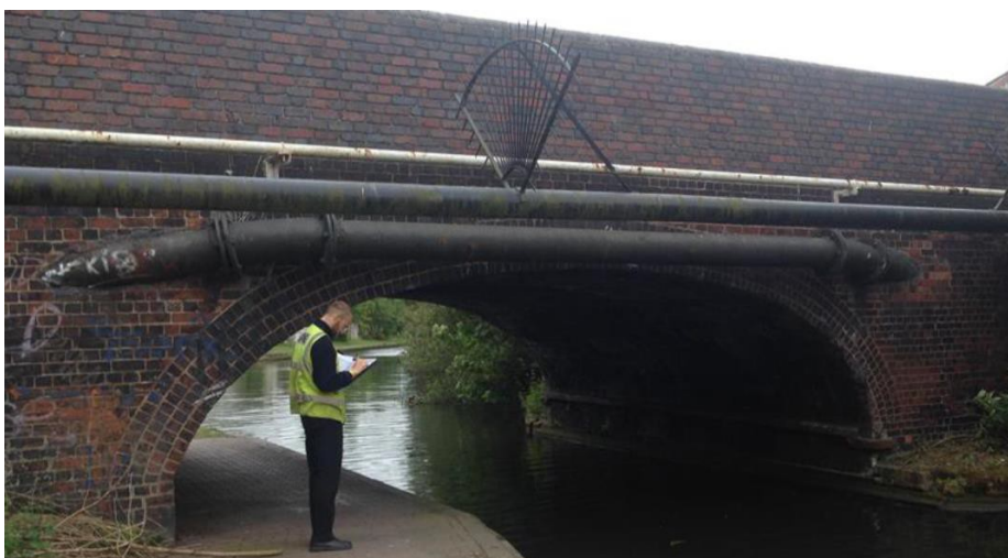
Figure 3: Pipeline crossing with unsuitable access deterrent measure
