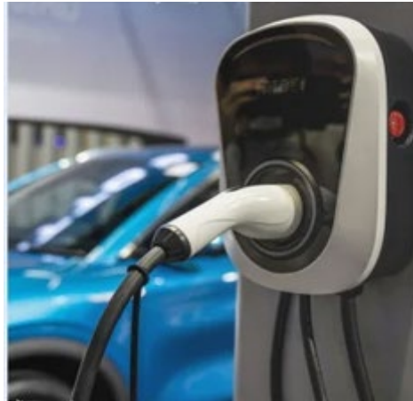
Figure 12: EV charging point
