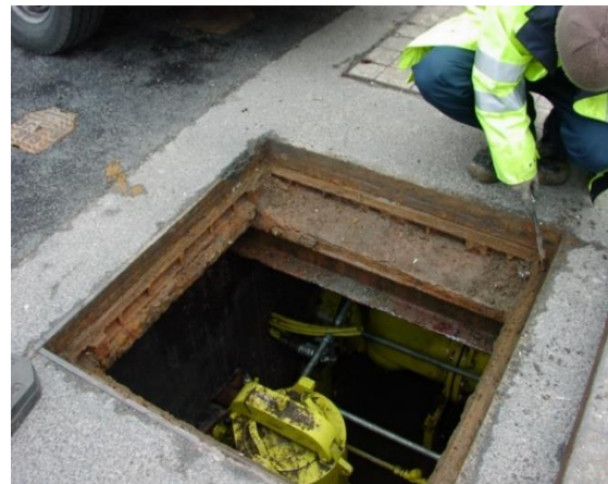
Figure 4: Donkin vector buried module containing an internal slamshut
