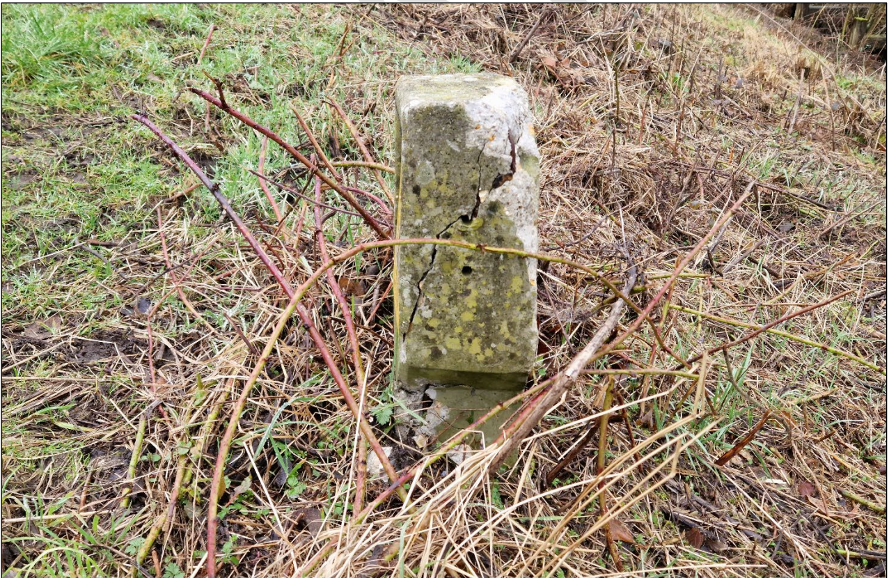
Figure 3-2 Damage to one of the CP posts containing the strain gauge connections, possibly caused by impact from cutting back equipment
