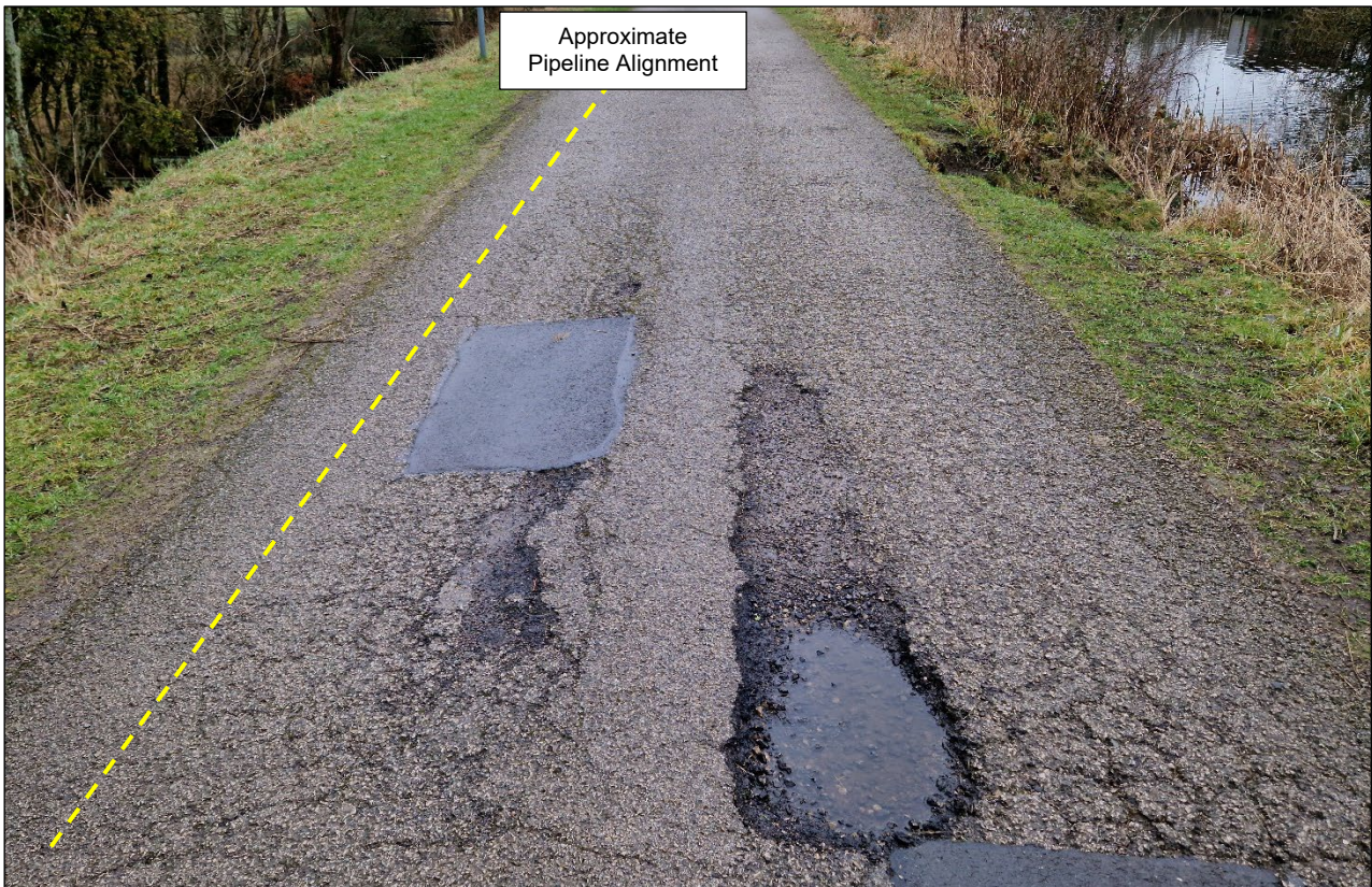
Figure 3-3 Evidence of continuing degradation of the road surface, including some surface depressions
