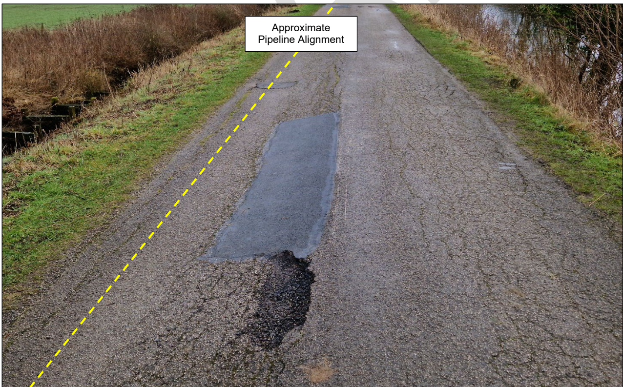
Figure 3-4 Evidence of continuing degradation and depression of the road above the pipeline
