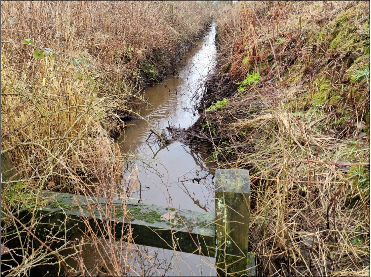
Figure 3-7 Section of propping missing, which coincides with where the slope “bulging” was observed (See Figure 3-6).
