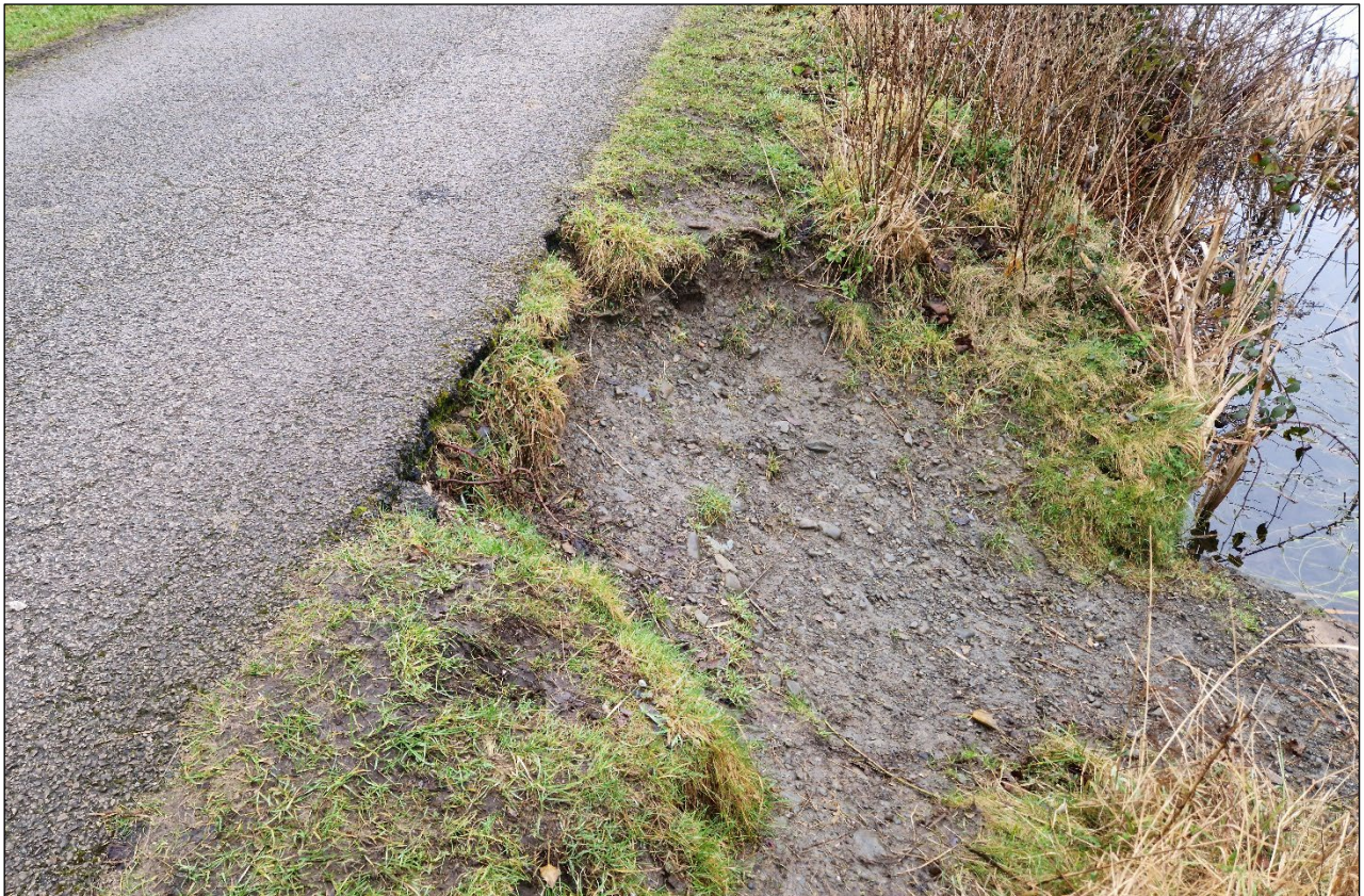
Figure 3-5 Evidence of damage to the canal side of the road, which could lead to further localised erosion and potential undercutting of the road
