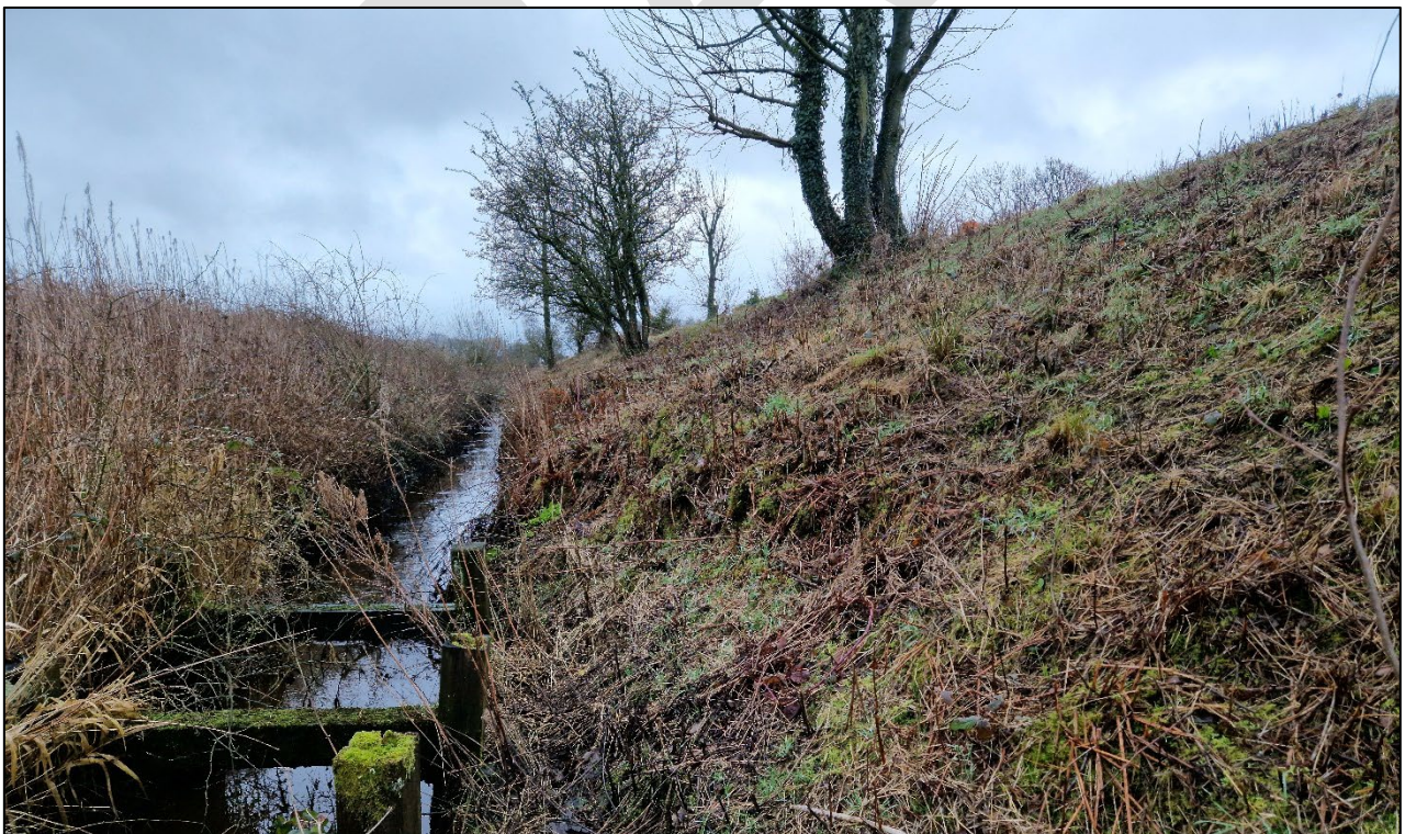
Figure 3-6 The northern slope (grassy area) appears to show bulging in a couple of locations, with possible identifying features of a slow-moving rotational movement at one location
