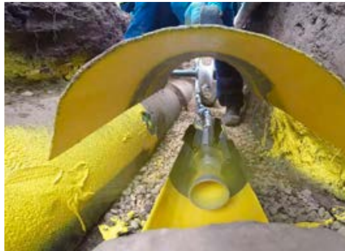
PRISM is a technique for spraying a liquid polymer inside the old cast iron main to create a new fully structural plastic main
