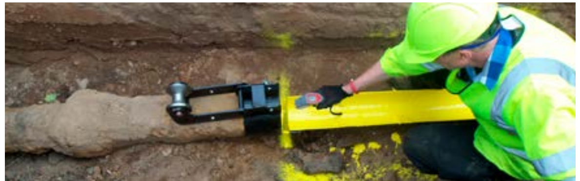
The stage gate process ensures projects are ready to move to the next level
