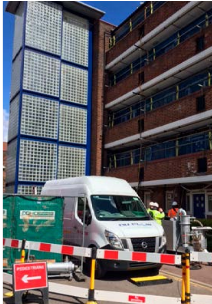
Repairing risers that supply gas to multi-occupancy buildings is a difficult challenge
