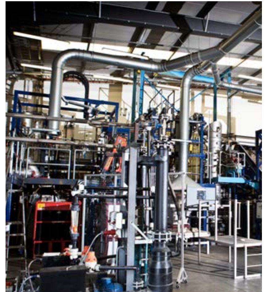
The BioSNG demonstration plant is a £23 million three-year project
