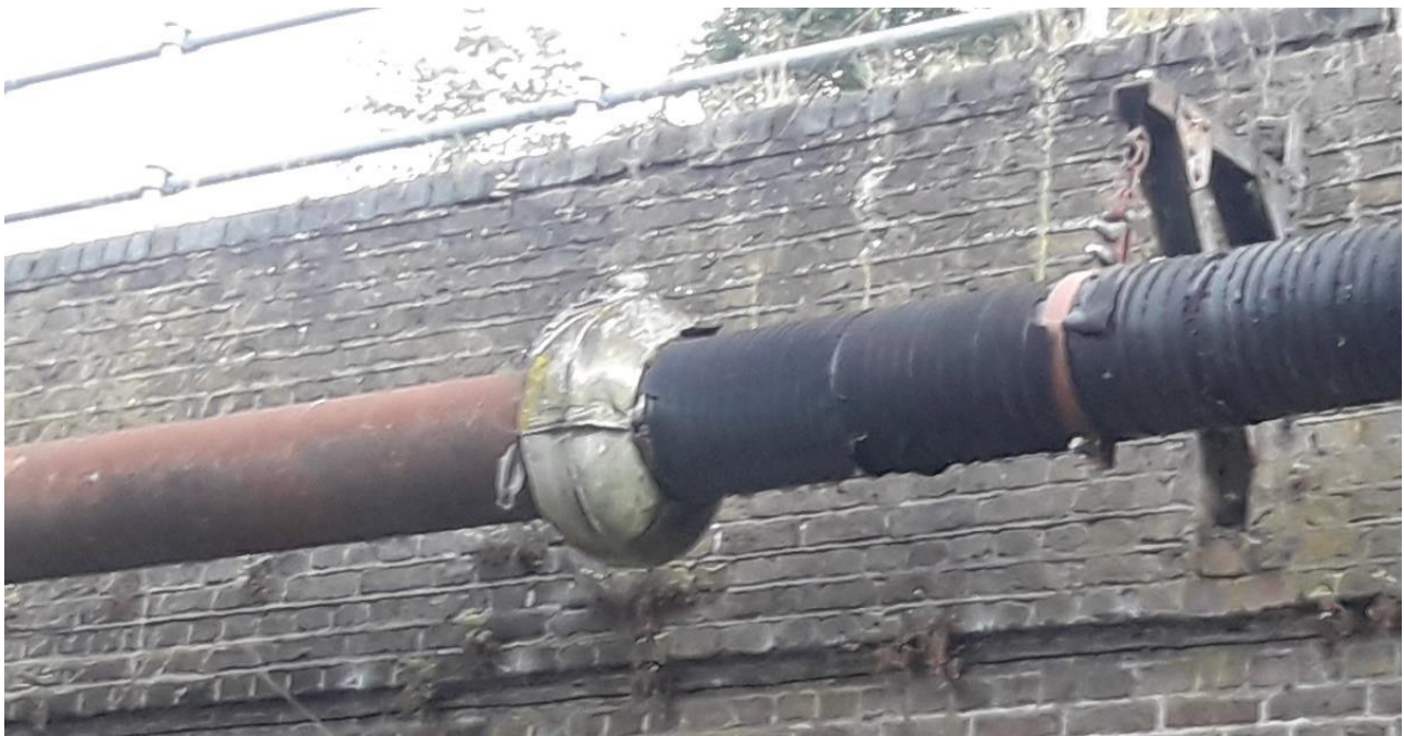
Figure 3: Typical pipe hanger & encapsulated flange on brick viaducts south of main bridge span
