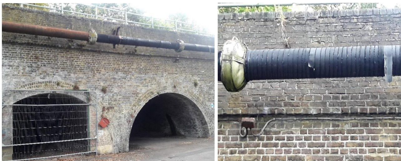
Figure 9: Part of tape-wrapped section
