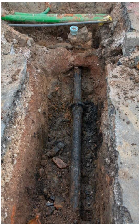
Picture 1: Example of a Cast Iron Main
