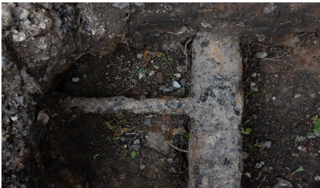
Picture 5: A Steel Service on an Iron Main
