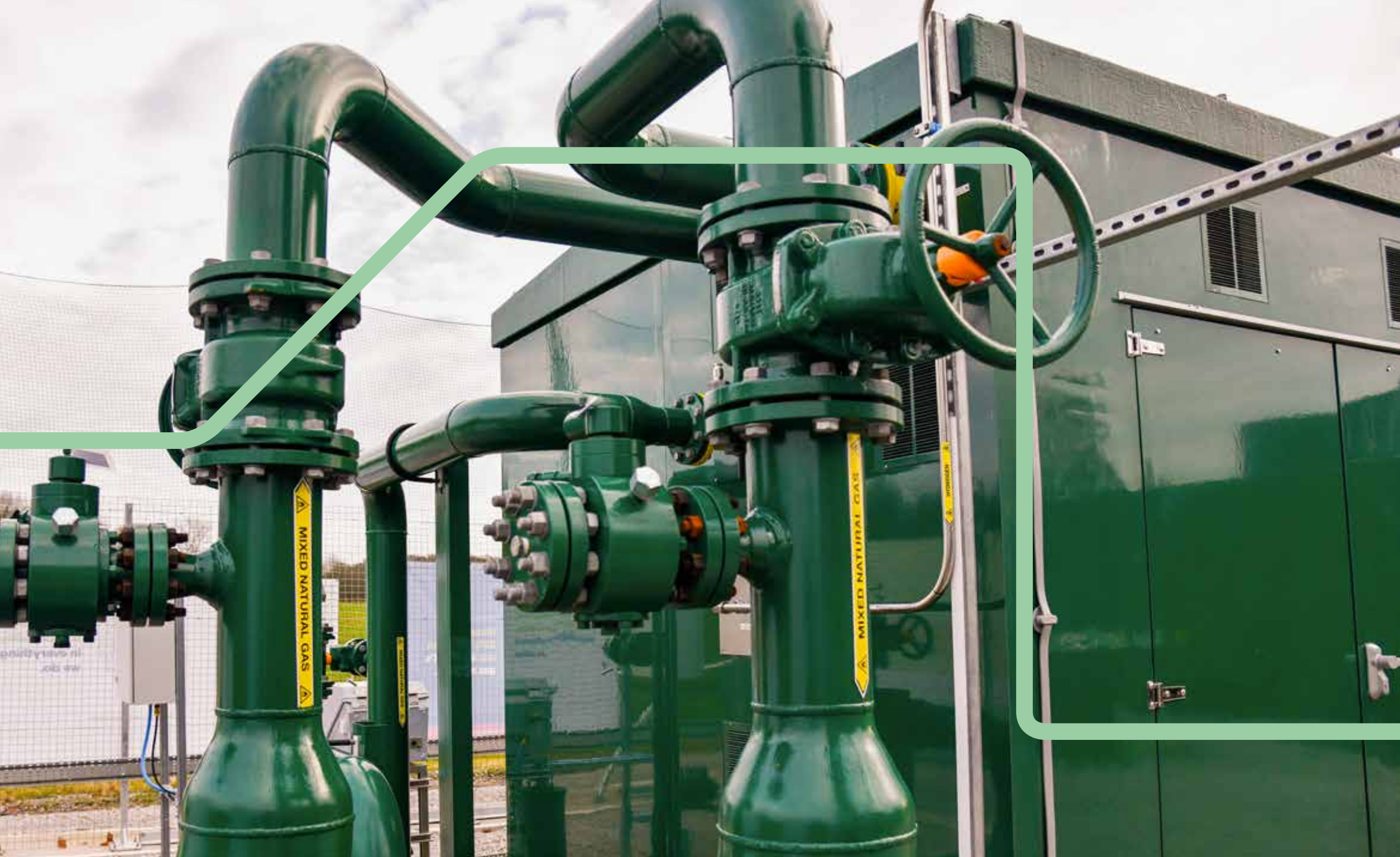
Above: HyDeploy at Keele University is a UK first.
