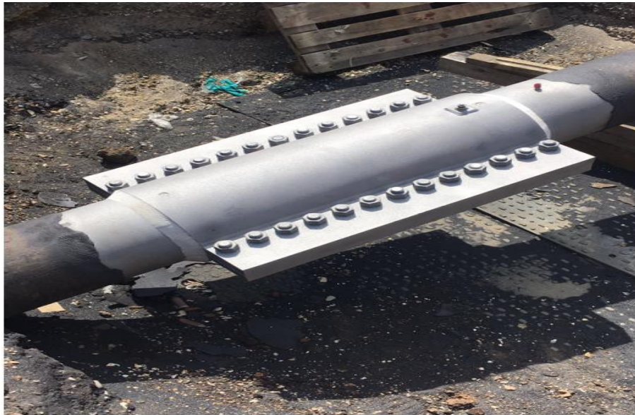
Figure 5: Corrosion example with repair clamp
