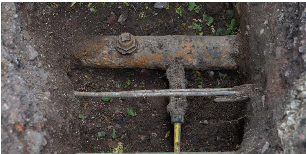
Figure 1: Yellow PE service tee off Steel mains
